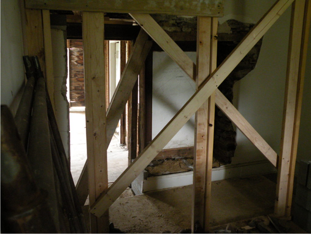
Plate 2 – Photo showing the location of the writing in the space of the former window on the north wall of the original stone section of the farmhouse. The door to the left of it gives entry to the addition brought to the farm possibly in 1865,
